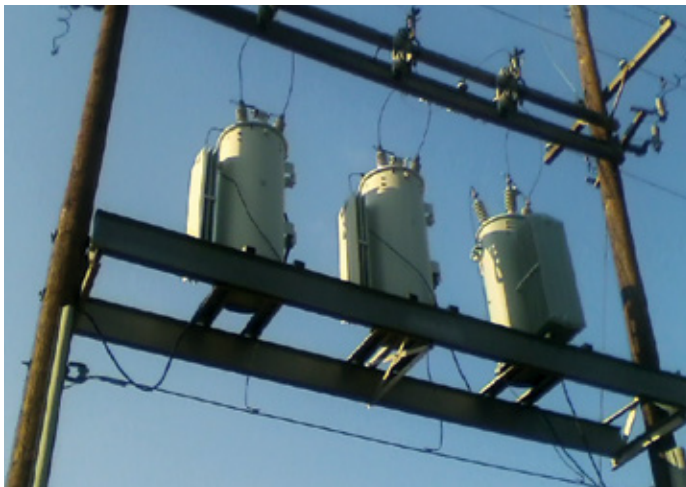
GE's Fast Cycle Voltage Regulator (VR-FC) installed in a distribution network
