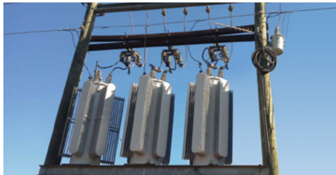
GE's Pole Mount Voltage Regulator (VR-PM) installed on a platform in a distribution network
