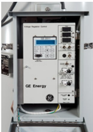
GE 2011B-E Controller Integrated in Flex-Connect Cabinet
